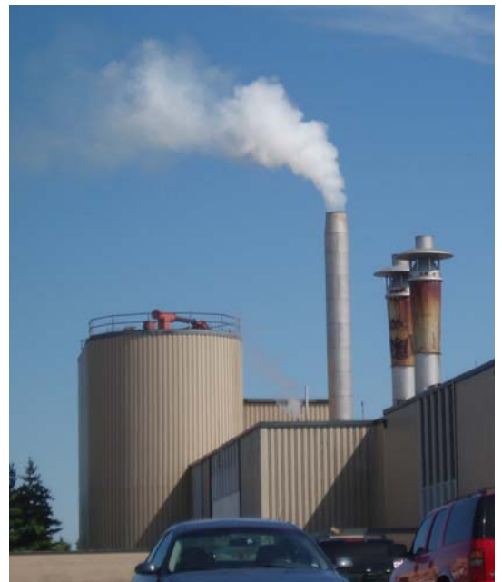
Wood storage silo and smokestack steam plume from the wood boiler at the Central Michigan University Heating plant
